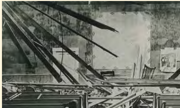
Interior of the Cherry Grove E.U.B. Church after the storm.
