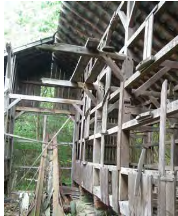
This interior photo from 2007 shows the post-and-beam structure of the crib, using one-inch in diameter hand-carved pegs.
