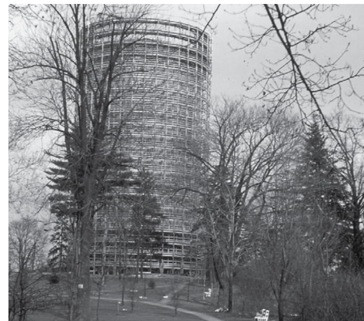
The Mt. Washington water tower under construction in 1939. It went into operation in 1940.
